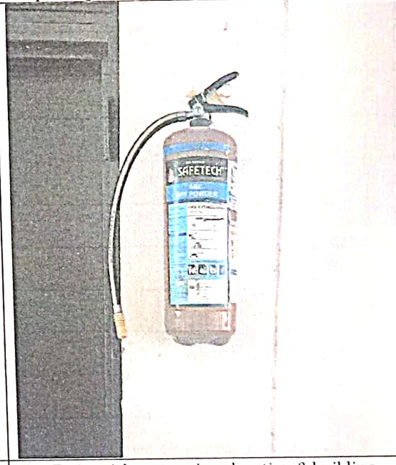
Fire Extinguisher at various location & building
