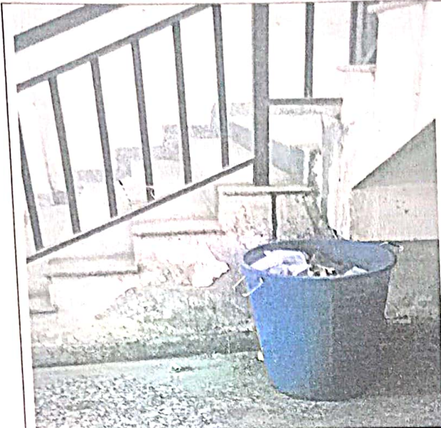
Bin provided for garbage collection
